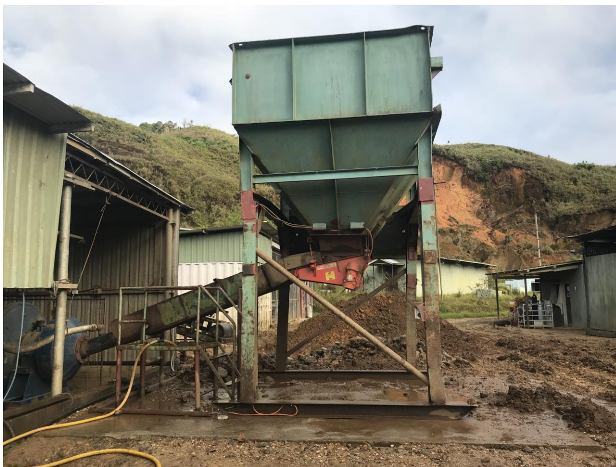
New vibrating feeder and feed shoot with stockpiled ore for the mill.
